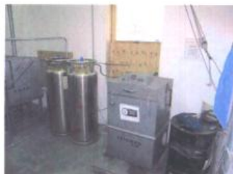
Deep-freezing unit for cryogenic treatment
